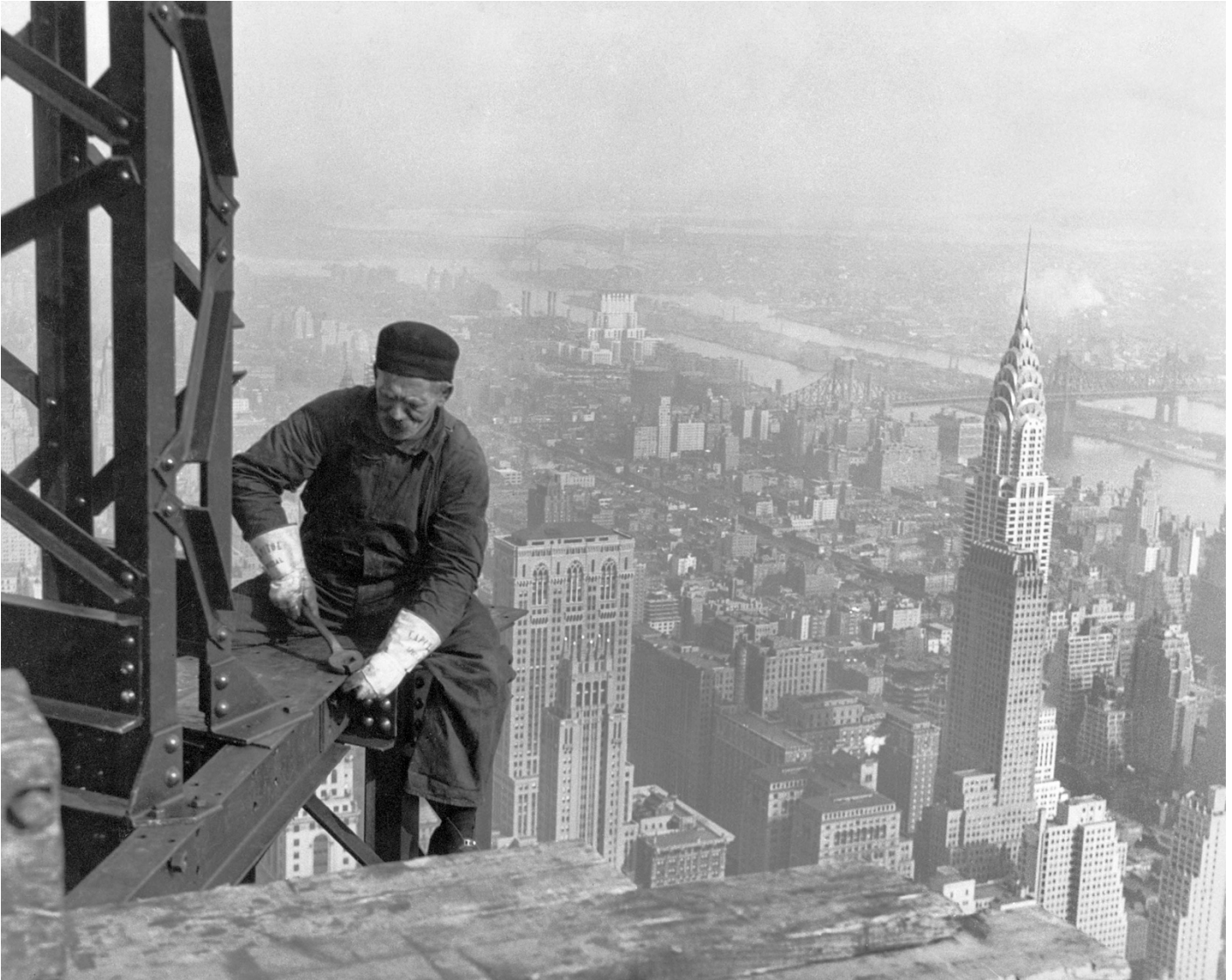
A worker adjusts a bolt on the Empire State Building, 1931. Photograph by Lewis Hine.
